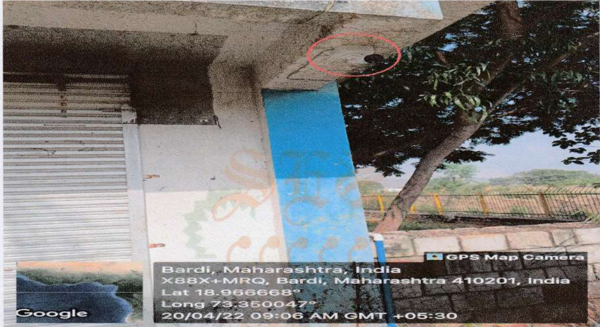
CCTV in main entrance
